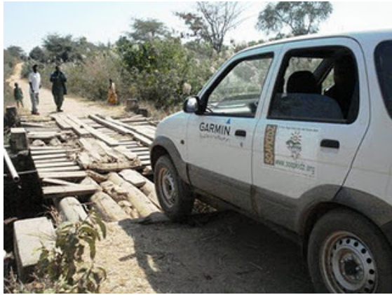
Another day, another bad bridge
